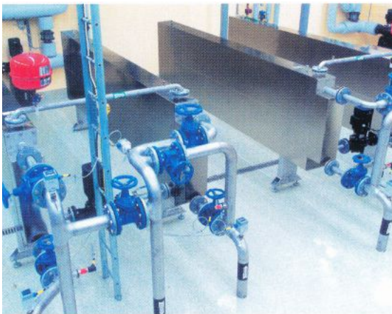
Two heat exchanger units sludge/sludge installed at Vimmerby wastewater treatment works in Sweden
